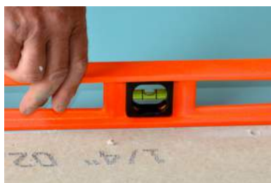
Make sure the shower base is level (bubble centered) all around. Check as you go.
